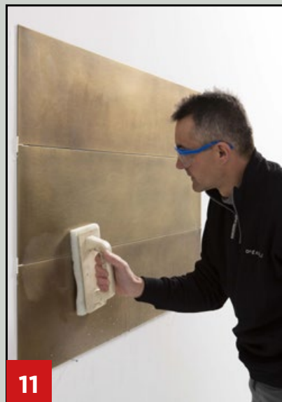
The “visible” surface of the slab must remain clean of adhesive residues. Immediately clean any residual glue that is still fresh with a rag.
